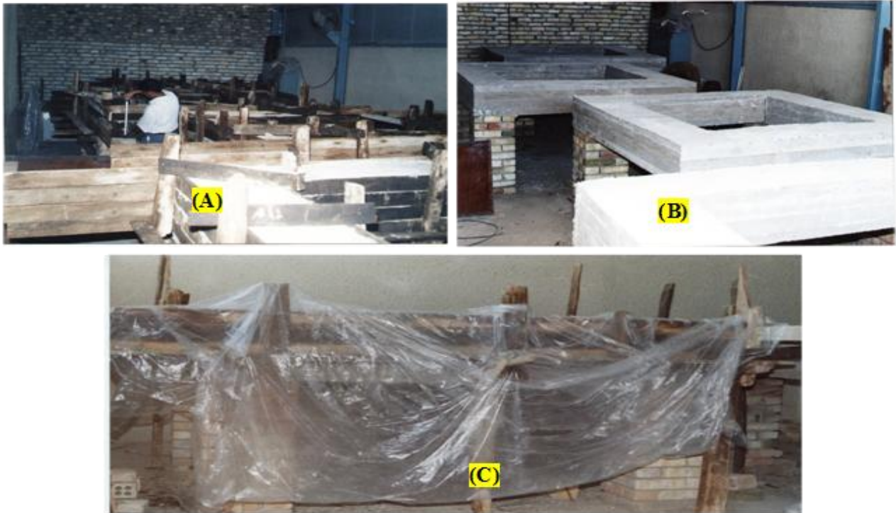
Figure 2. (A) The wood formwork of the rigid beams; (B) The rigid beams after lifting of the wood formwork; (C) Curing of Rigid beam with the wetted hessian and polythene sheets.
